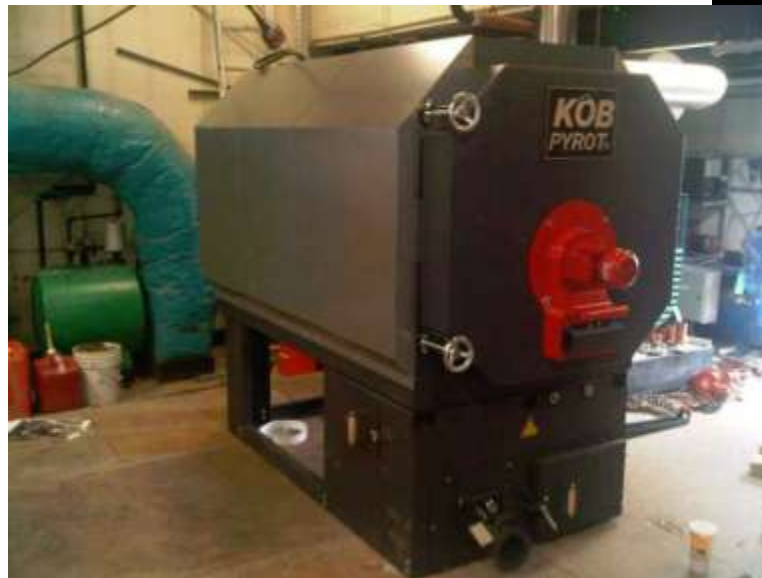
Wood Pellet Boiler
